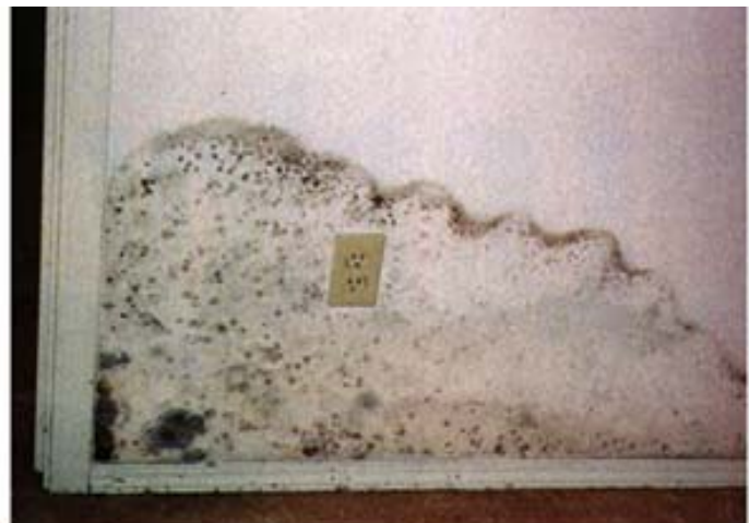
Mould growth on the interior surface of gypsum board resulting from high moisture content in the exterior wall assembly.
