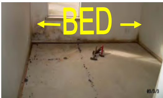
Figure 8 Mould on Interior Surface of Exterior Wall in Bedroom
