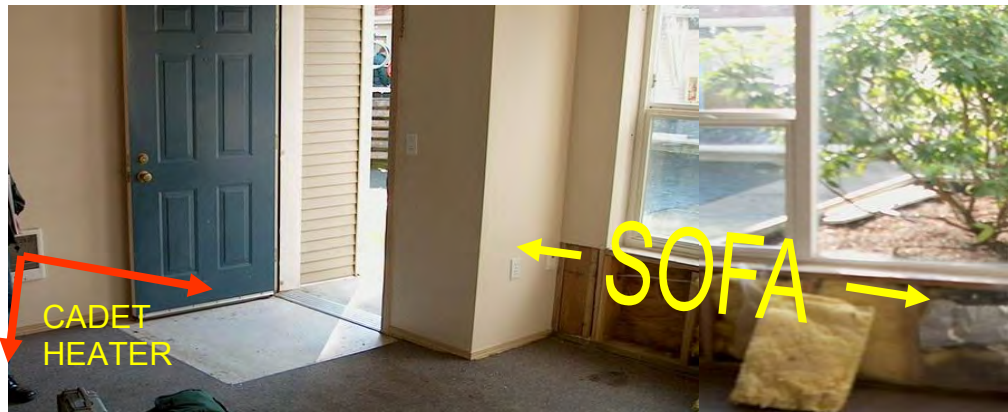
Figure 10 Location/Orientation of Cadet Heater, Furniture and Resultant Mould
