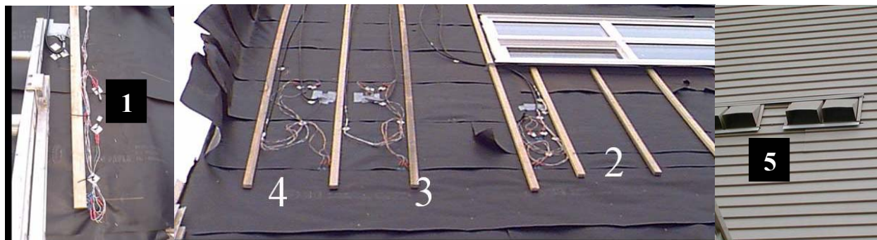
Figure 2 – Cavity Locations, Building 1 (1-Balcony saddle, 2-Window Corner, 3- Control, 4- Electrical Box, 5- Dryer Vent)
