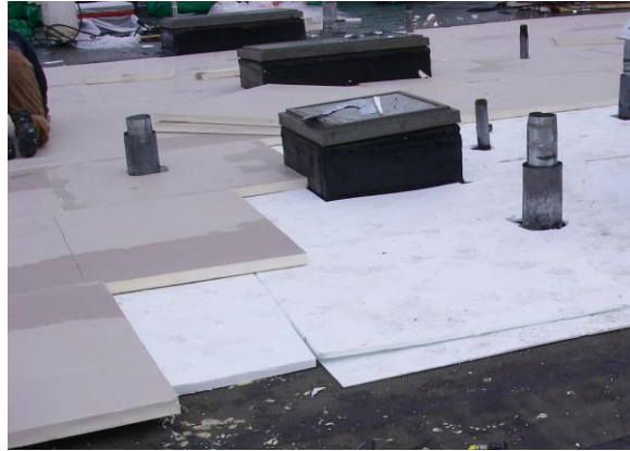
Figure 1: Tapered EPS insulation below polyisocyanurate insulation in a low slope roof application.
