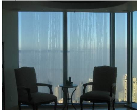
Figure 8: Severe condensation and frost inside glazing unit during cold weather.
