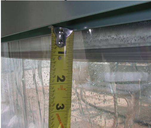
Figure 7: Spacer bar displacement into glazing unit obstructing view and resulting in fogging.
