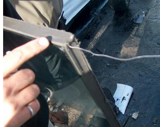
Figure 10: The culprit: unsealed vent tubes. The solution: crimp and seal them.
