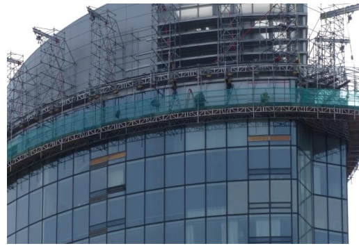
Figure 2: Glazing replacement project at a 45 storey high-rise building utilizing a large suspended stage hung from the building
