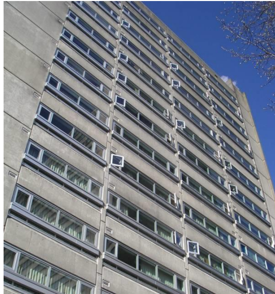
Figure 1: Is the Argon gas fill that we specified actually present in these new windows?
