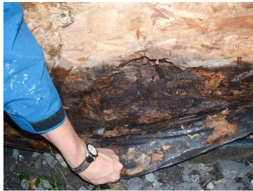
Figure 3: Adhered membrane base flashing restricts drying
