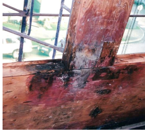
Figure 5: Decay worse under membrane location
