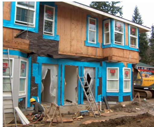
Figure 6: Extensive use of self adhesive membrane results in almost complete coverage of wall area on ground floor of this building.
