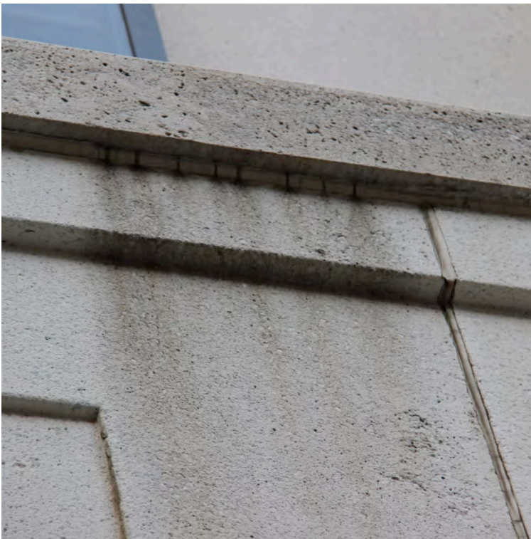
Figure 16: Drainage without weep holes. The horizontal sealant joint in the photo to the left is cracked and allows water to drain from underneath the window sill above. This is not a planned drainage path.
