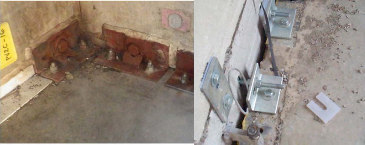
Figure 11: Panel attachments at a typical exterior corner. For the structural system, the inspection should include a visual inspection of all structural components by a structural engineer experienced in the design and construction of precast concrete structures. This connection, photo on the left, is not well protected from corrosion, and hence would require more frequent inspections than the industry recommended hot-dip galvanized connection seen in the photo on the right.
