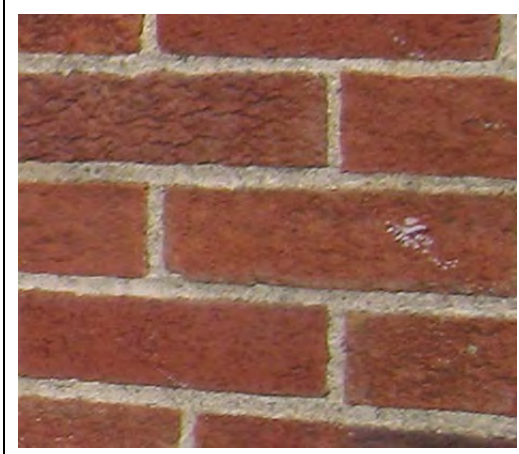
This wall has been exposed to water and multiple freeze-thaw cycles, but shows no sign of damage.
