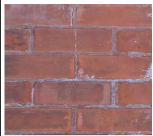
This wall looks fine, but later became badly damaged when it was exposed to more water.
