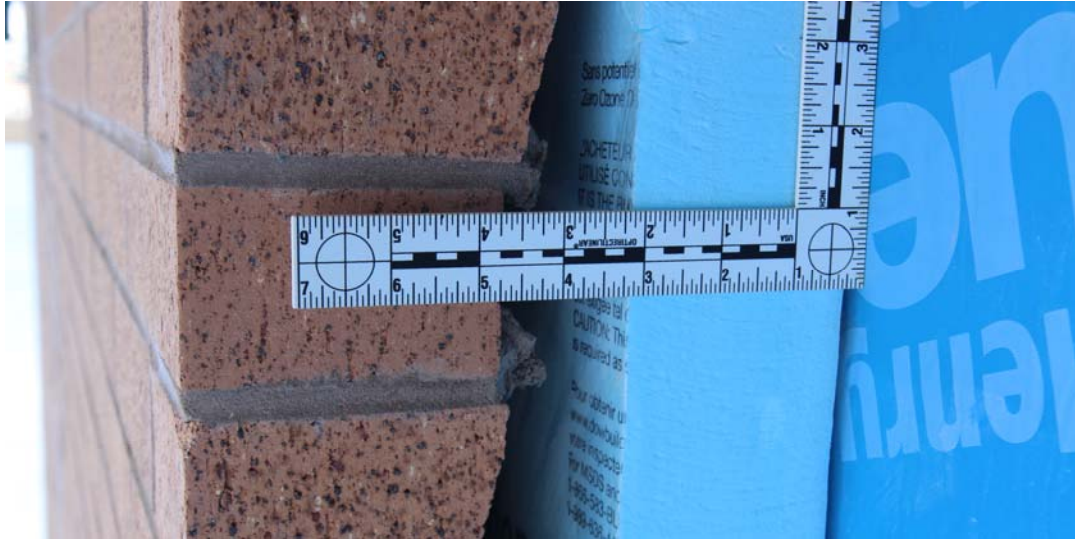
Figure 8: Actual air gap (1/4" or 6 mm) measured behind insulation on a school enclosure
