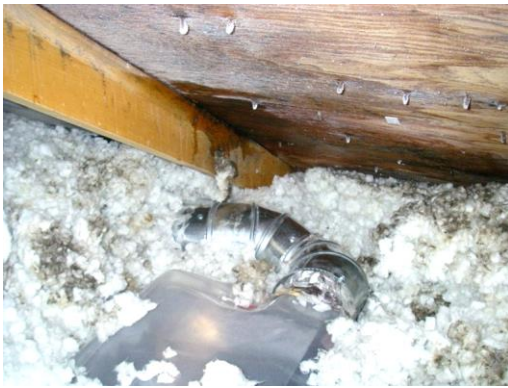
Figure 1: Locally stained and wet sheathing due to condensation (frost) of humid air which is leaking from a poorly sealed bathroom exhaust duct
