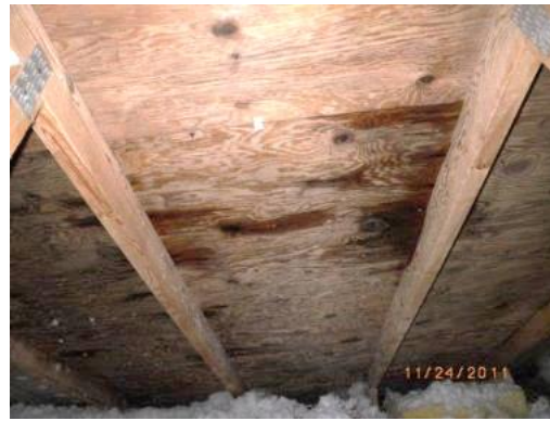
Figure 2: Visibly wet roof sheathing caused by rainwater ingress through the shingles and underlay
