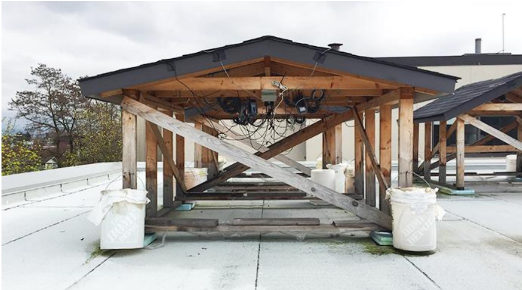
Figure 3: Roof hut decoupled from interior conditions by unrestricted ventilation to the underside of the roof sheathing. Monitoring equipment was installed to measure performance characteristics including sheathing moisture content at various depths, roof surface temperature, sheathing temperature, and ambient temperature and relative humidity.
