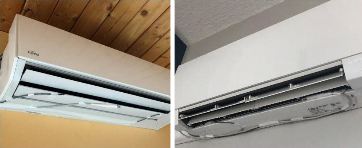
Figure 3.31 – two different strategies for mounting supply temperature sensors: adhered to oscillating louver (left – PRI01i) and adhered behind the louver (right – KEL01a).
