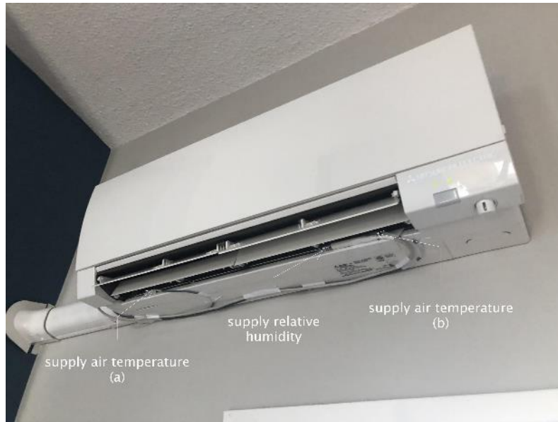
Figure 2.5 - indoor unit with temperature and relative humidity sensors at supply louver (bottom of unit).
