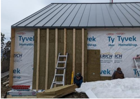
Figure 10: Exterior insulation was installed over a water-resistant barrier (WRB) on the case study building. The WRB is the last line of defence to water penetration in the wall assembly.
