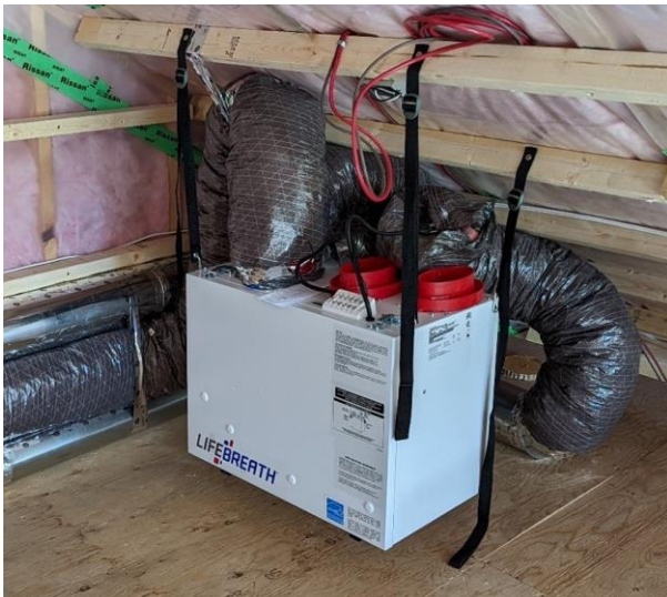
Figure 12: The high-efficiency, fully ducted ERV installed in the case study home.
