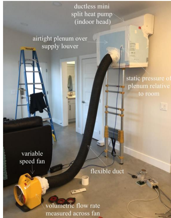
Figure 2 Volumetric flow rate measurement configuration for ductless indoor units.
