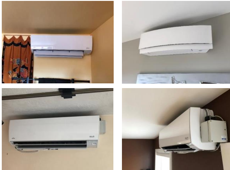
Figure 4 Ductless indoor units with limited ceiling clearance.
