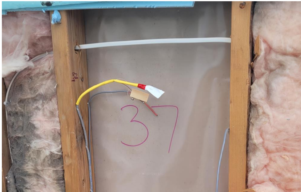
Figure 11: A relative humidity, temperature, and wood moisture content sensor to be installed between the fiberglass batt insulation and the exterior EPS insulation of Unit 37.
