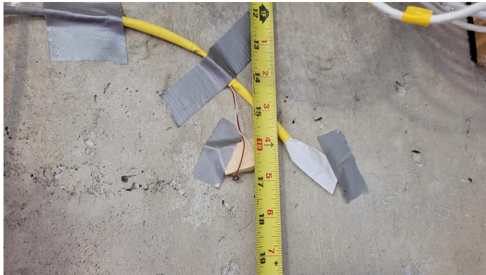
Figure 12: Enclosure moisture monitoring sensors installed against the concrete wall prior to spray foam application.
